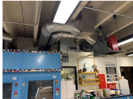
Photo 4 – Exhaust Hood with Make-up Air Fan
