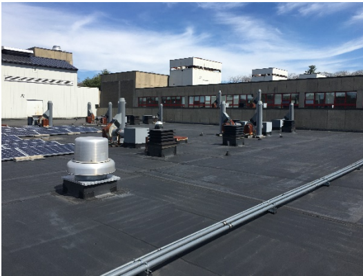
Photo 3 – Rooftop Exhaust Fans
