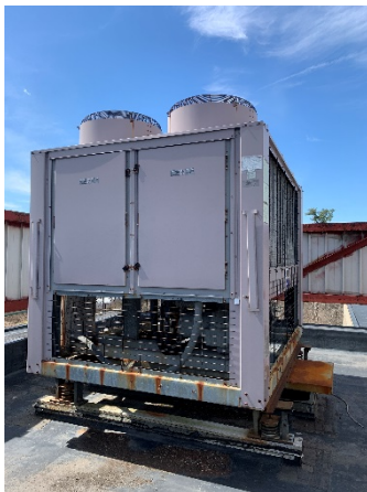
Photo 5 – Air-Cooled Condensing Unit
