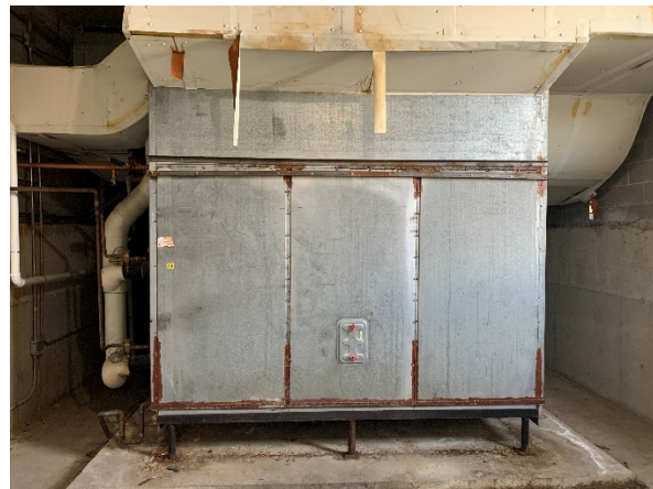
Photo 6 – Penthouse Air Handling Unit
