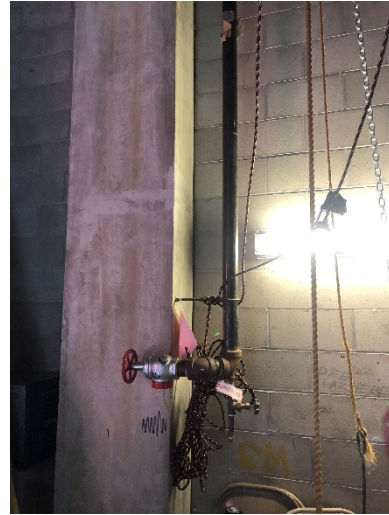
Photo 2- Stage Hose Connection
