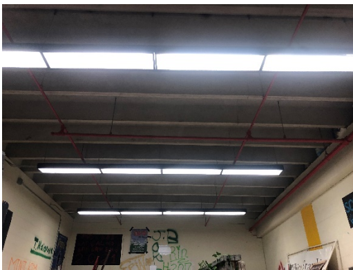
Photo 3 – Storage Room Sprinklers
