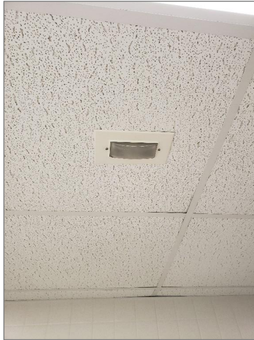
FIGURE 17: VISUAL ALARM NOTIFICATION DEVICE IN RESTROOM
