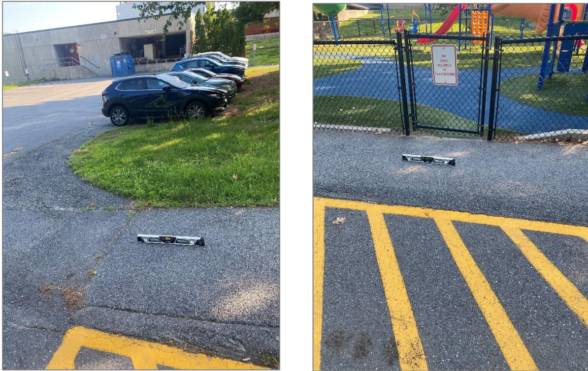
FIGURE 6: EXTERIOR ROUTE DEFICIENCIES
